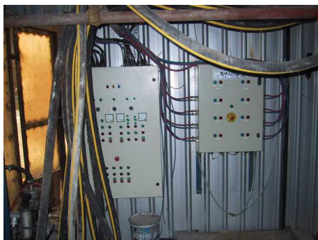
Control Panel & Hydro-Pneumatic Control
