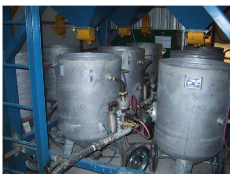
Blast Pots installed under Abrasive Tank
