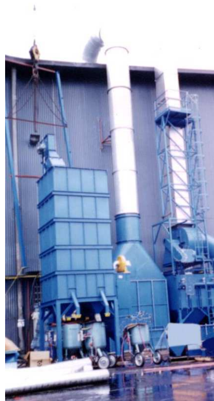
Abrasive Tank, Paint Booth & Dust Exhaust Elevated Inspection Platform Roof Shed Installation in Progress for Tank
