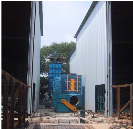
Equipment Between 2 Chambers
