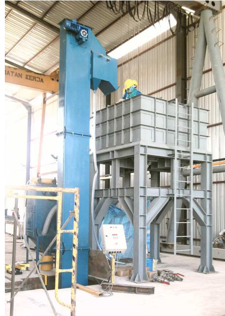
Typical Recovery Bucket Elevator, Separator & Tank used in Small Blast Chamber
