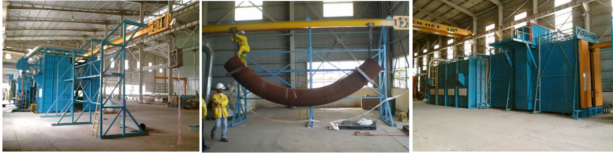
Monorail Hanger at Loading Bay, Loading Long Radius Pipe Bend, Going Through Blast Room & Heating Oven
