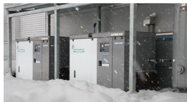
Manufacturing plant: SMS15SD x 2
