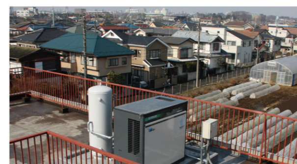
Component manufacturing plant: SMS11ED x 1
