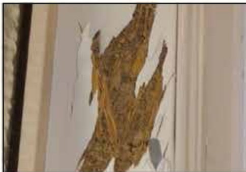
Damage to house
