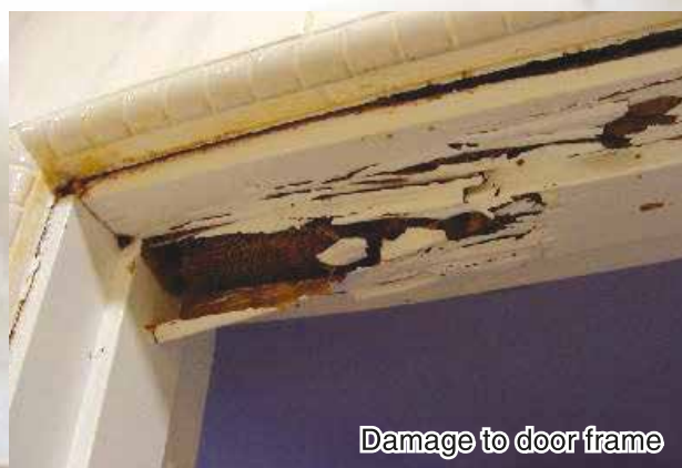
Damage to door frame
