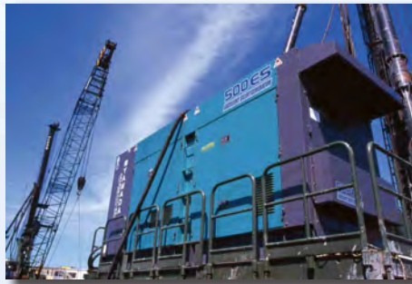
As the power source in the construction site.
