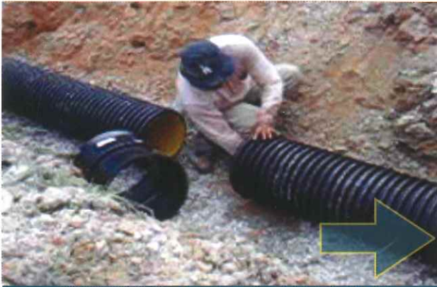
Clean pipe ends, rubber rings and internal faces of the socket with soap water
