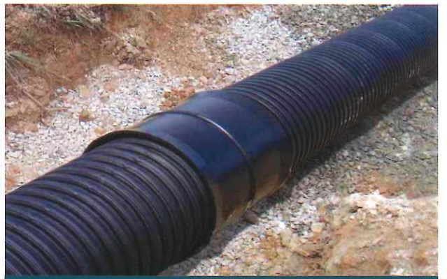
Push socket into pipe carefully, ensuring that the socket ends are protected from damage
